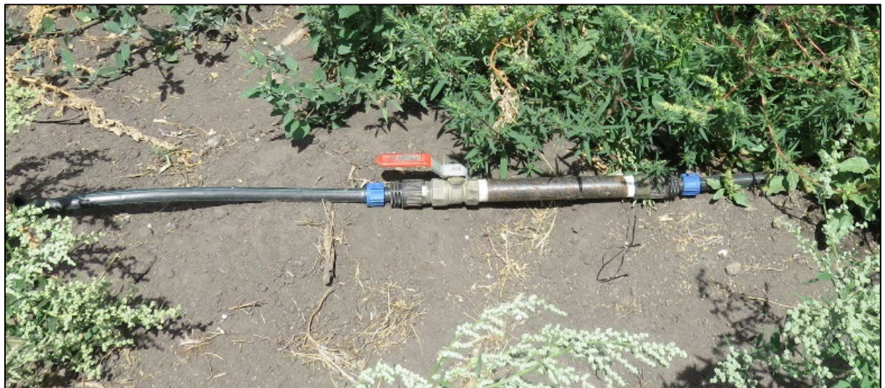
Photo 7: Example of a shut-off valve for an irrigation system on a newly planted tree belt.
